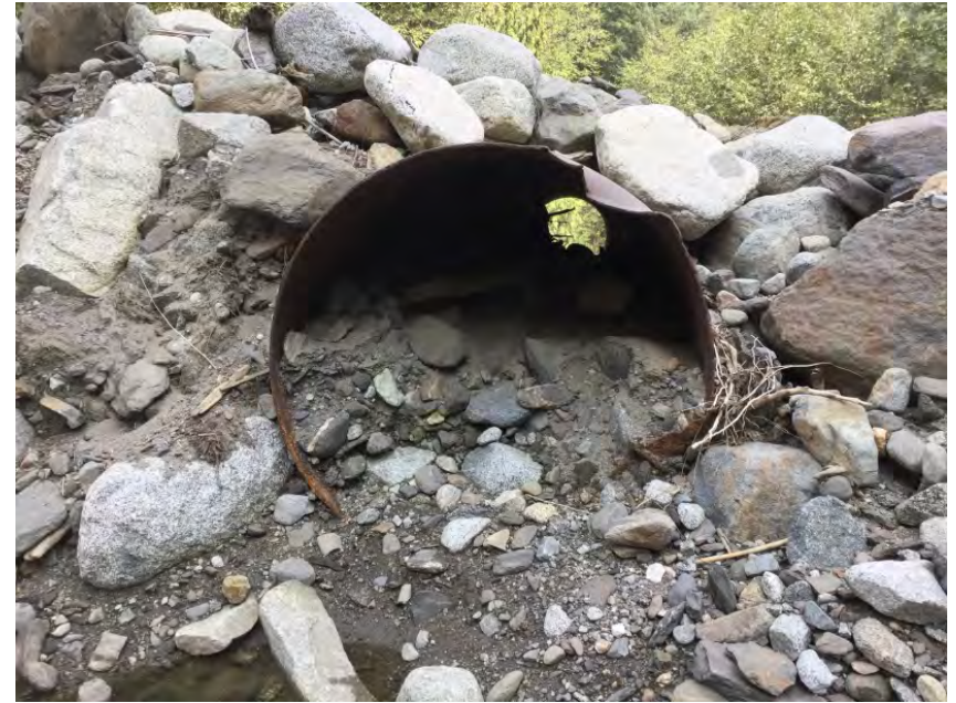
Right culvert 50% plugged
